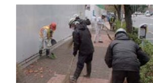
Cleanup activity at the "Shibaura 2-chome, Minato-ku New Construction Project (tentative name)"
