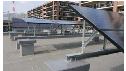
Solar Photovoltaic Power Generation Panels
