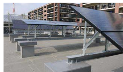
Solar Photovoltaic Power Generation Panels
